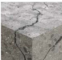
Cracked concrete C20/C25 to C50/C60
